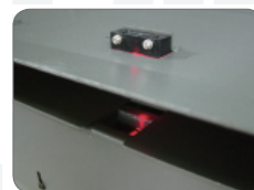
Fire protection sensor
